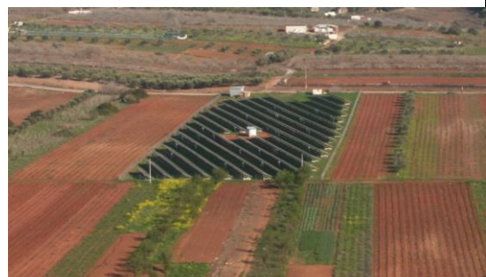
Figure 30b PV-Panels in parallel to the airstrip of Athens Airport. This can be considered as best practice as the installation respect at best the already given rectangular layout of infrastructure and agriculture. (Photos: Alexandra Kruse 2017)
