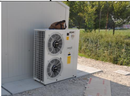
Figure 21a Air source heat pump, Ferrara. (Photo: M. Bottarelli 2017)
