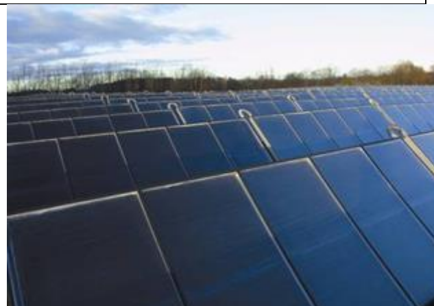
Figure 26b Type b) Solar Thermal Collector field on the ground. (Photo: ARCON/ESTIF 2016)
