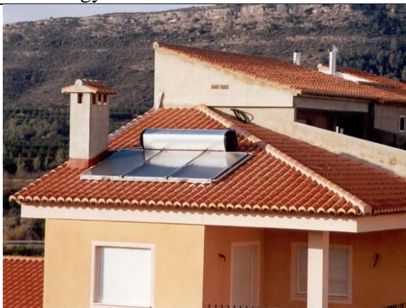
Figure 26a Type a) Domestic Solar Hot Water System on the roof of a building. (Photo: Solahart/ESTIF 2016)
